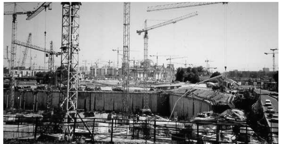
East Berlin - the largest construction site in Eastern Europe, (Photo Courtesy of Jasen Higgs)
