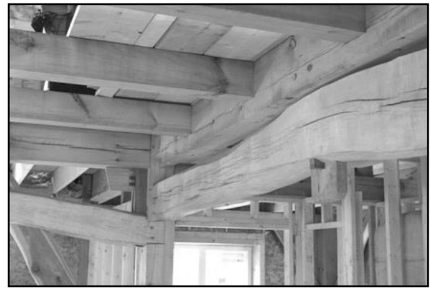
Two locally sourced timbers are used to replace a larger timber not available near the site.
