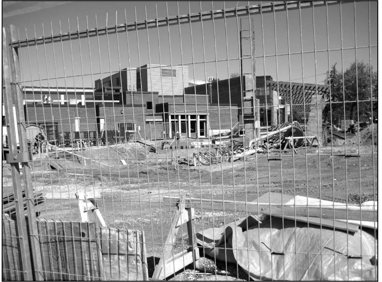
The Bomber Patio is currently closed for business as construction continues to extend service tunnels from the SLC to Biology 2 to set way for the construction of the Quantum-Nano Centre on the B2 Green. The original schedule had called for the extension to be finished by this month.
