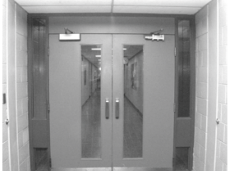
Double doors are found around much of the campus and require special attention
