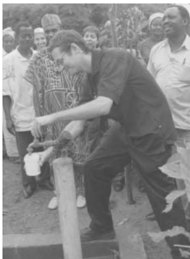
EWB overseas volunteer Ian Randall draws the first water from a new well in Bapa, Cameroon.
