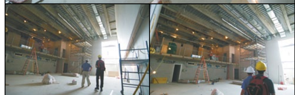
The expansive multipurpose room which can hold large seminars or events. The upper balcony can be separated to hold smaller events if needed.
