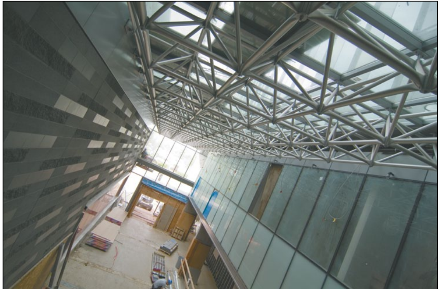
The main entrance foyer of QNC. Visitors will be able to see the cleanroom on their right hand side upon entering from Ring Road
