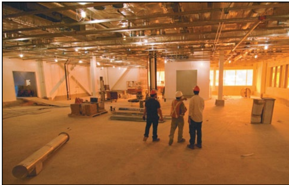
The cleanroom within QNC still under construction. The orange glow is due to the tinted glass which filters certain wavelengths of natural light.
